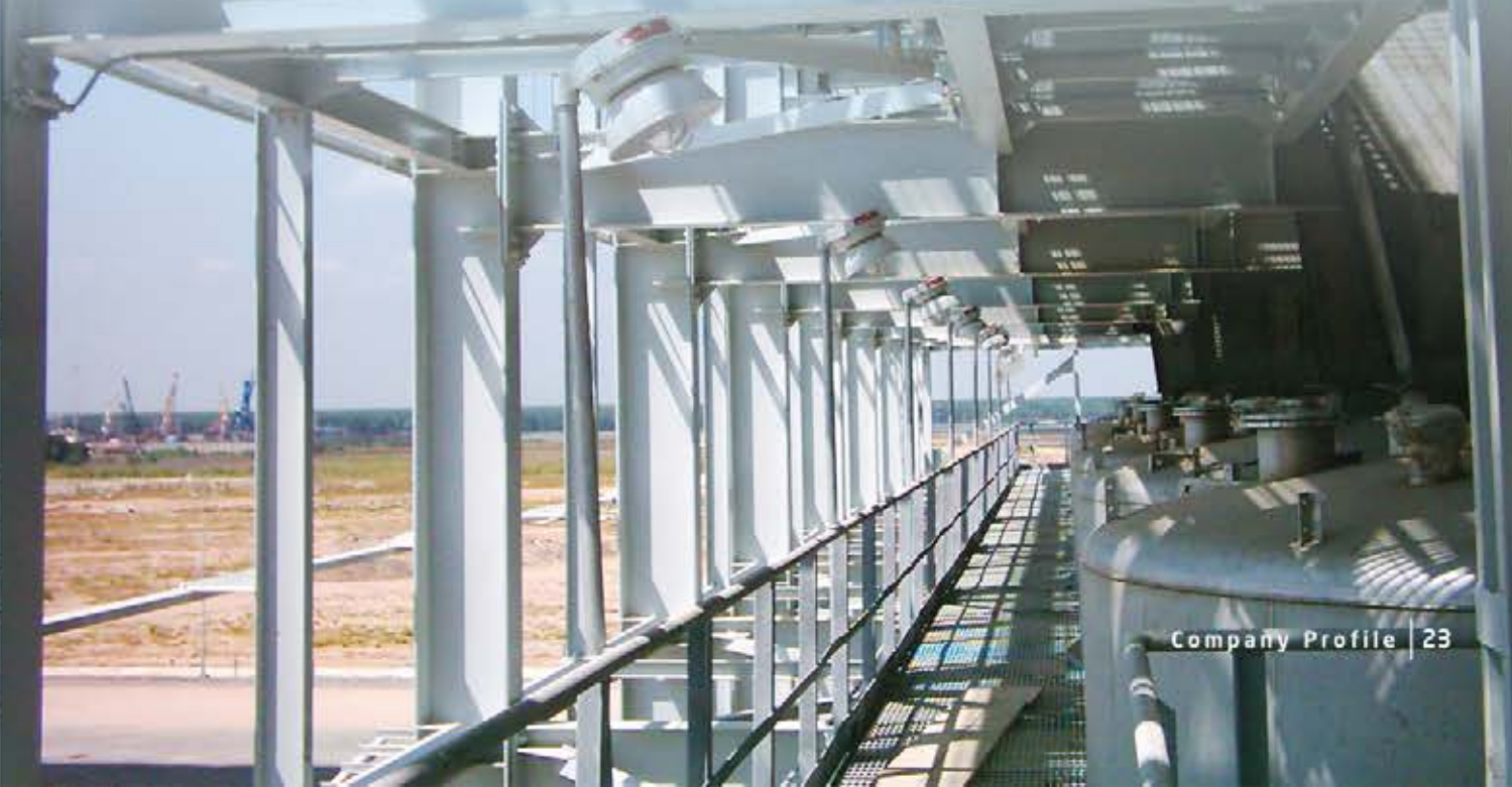
HAZARDOUS AREAS - LIGHTING SYSTEM
