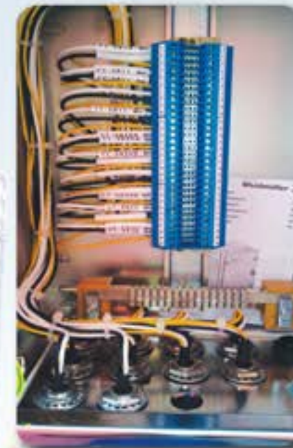
TERMINATION OF JUNCTION BOX
