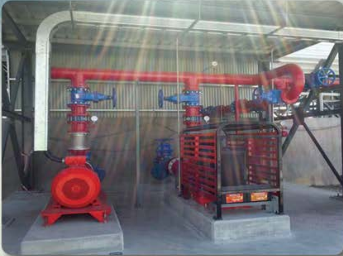
FIRE PUMP STATION
